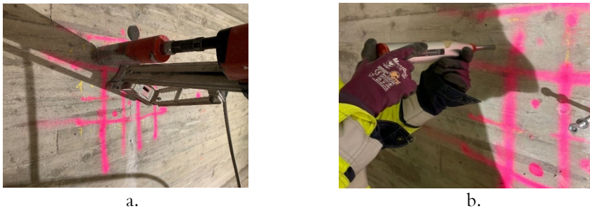
Figure 25. a. Drilling of concrete cores and b. concrete strength test with Schmit hammer.
